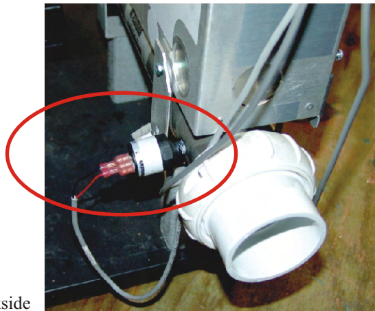
Pressure Switch Location
