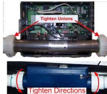
Figure 17 - Unions Tight (Balboa – Above Top; IN.PL – Above Bottom)
